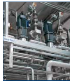
CR pumps installed in a dairy plant
