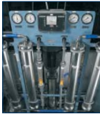
CR(N) 5 installed in a water treatment plant
